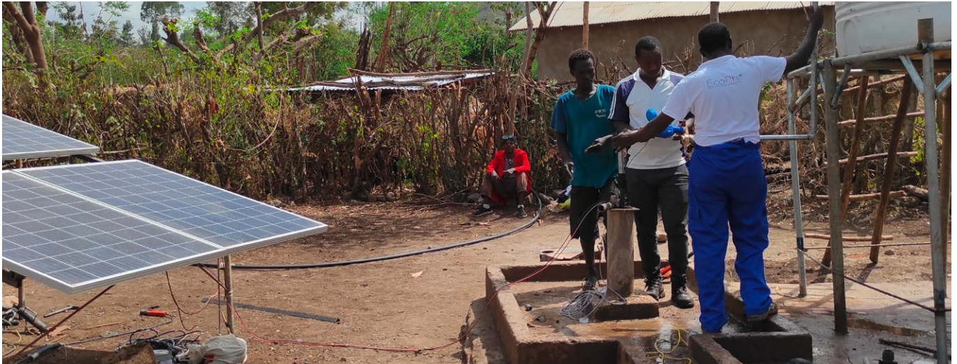
Systems by EcoPhi help a rural community better monitor the PV water pump
